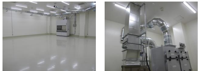
Figure 2 Beryllium facilities (beryllium room and ventilation system)
