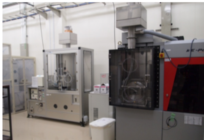
Melting (left) and sintering (right) devices installed in the Beryllium Handling Room.
